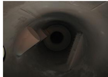
Inspection area #6: The exh. receiver was found clean and no signs of unburned fuel / deposits.
