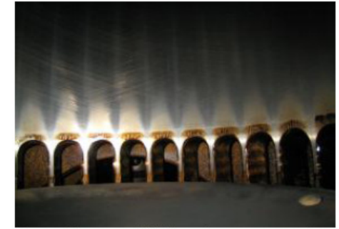
Inspection area #5: The piston crown and ports were found without any deposit.
