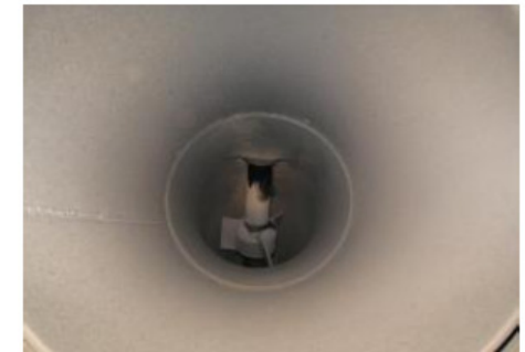
Inspection area #7: The exh. valves were found in good condition. During previous dismantling of exh. valves, some major deposits has been found in the seat area.
